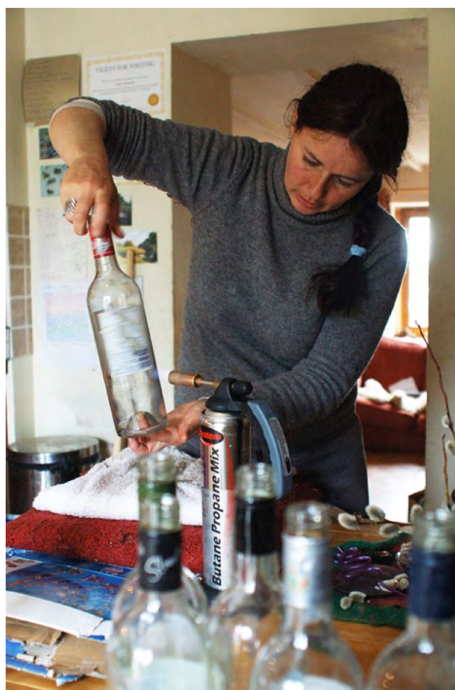
Hoppie cutting old wine bottles into glass bricks for use in the construction of a wall in her eco-house
